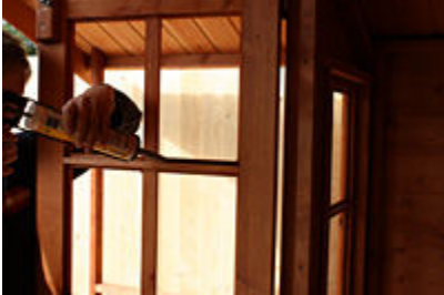
31.Photo,32.Photo Glazing. With the silicone apply a continuous bead round the rebate and centre spar
