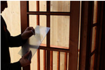
33.Photo Peel of the protective skin on both sides of the polycarbonate pane.
